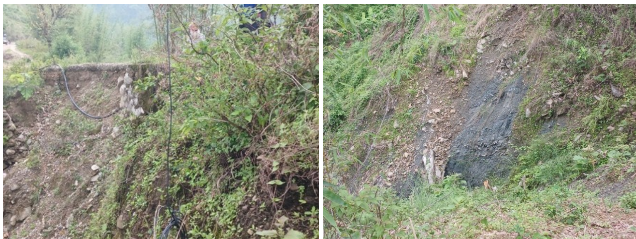
Photograph 49 Landslide Site, Lamitar
