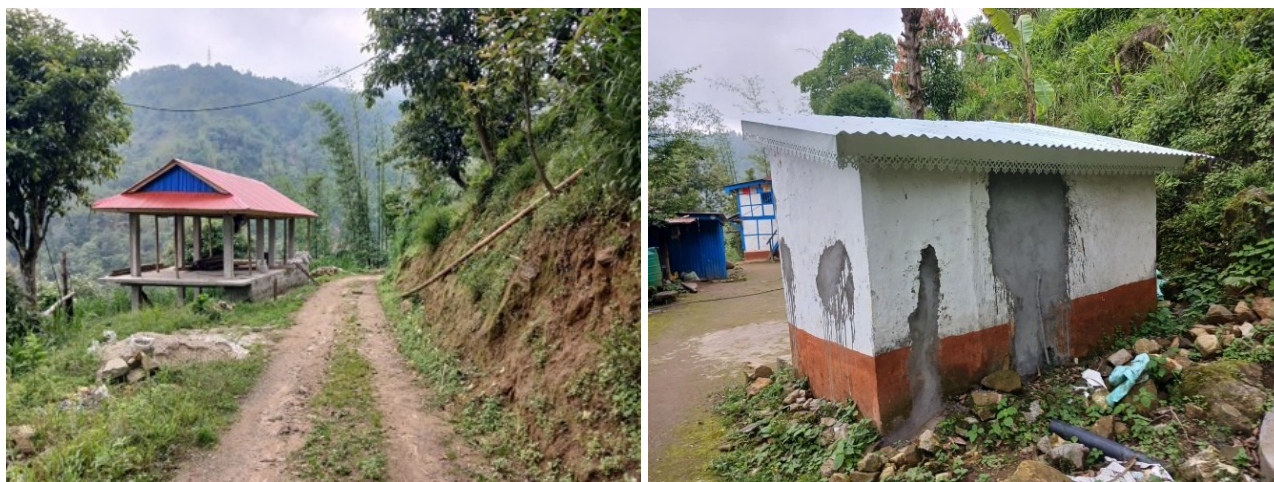
Photograph 52 Landslide Site, Maidane
