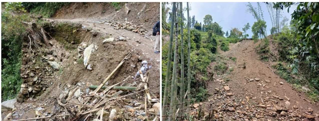
Photograph 19 Landslide Site, Bhalukbola/Thalukbola Khand
