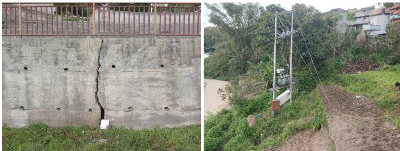
Photograph 53 Landslide Site, Tudikbel (Mathillo Kopche) Parbat District
