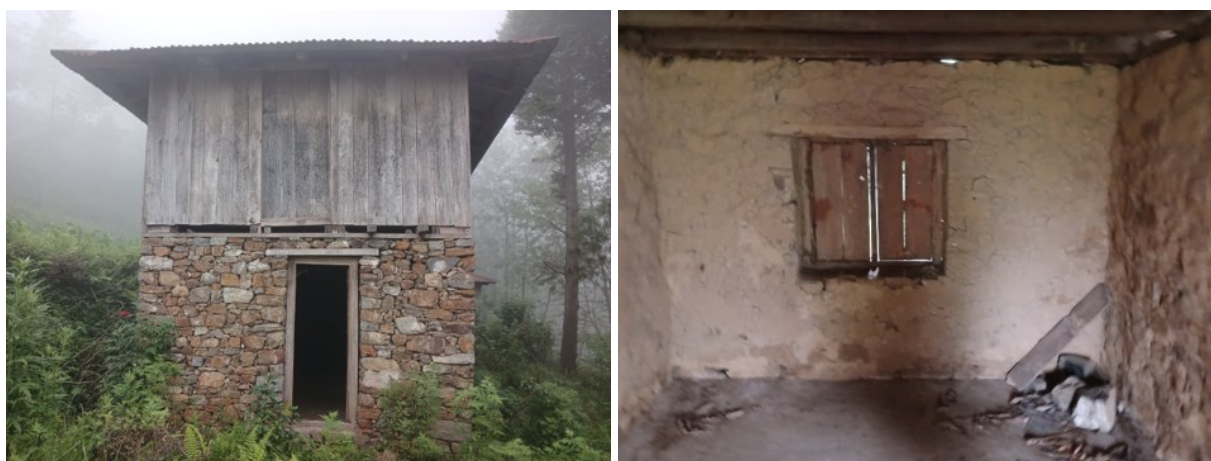
Photograph 35 Landslide Site, Doctor Gaun Kolbote Tol
