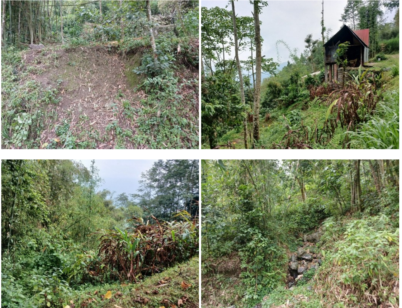
Photograph 33 Landslide Site, Triveni Tol
