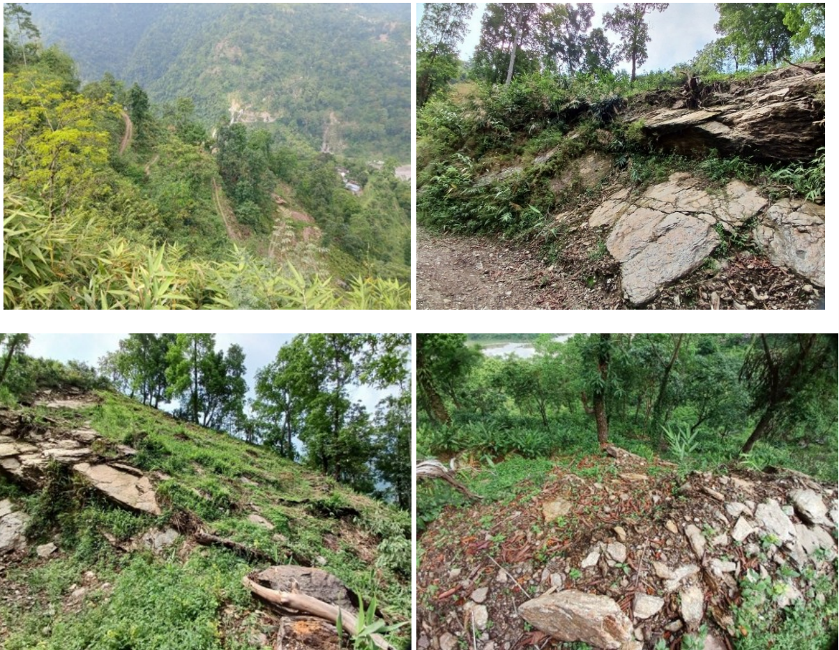
Photograph 21 Landslide Site, Ambitar
