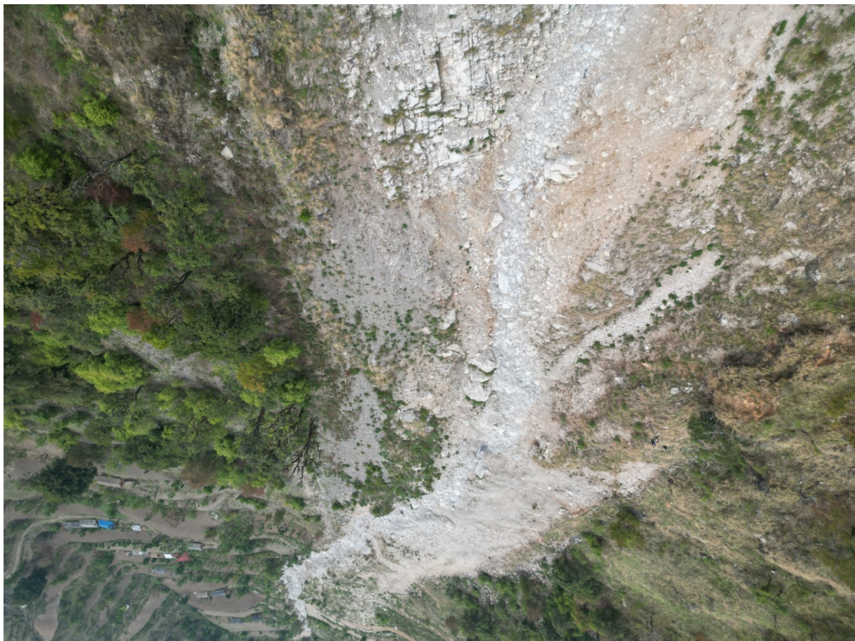
Photograph 61 Landslide Site, Kalo Pabiro
