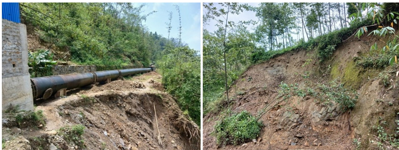
Photograph 47 Landslide Site, Gumba
