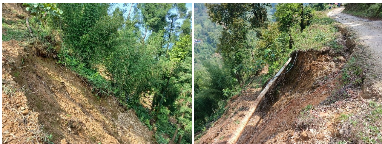
Photograph 13 Landslide Site, Mayukhola Area
