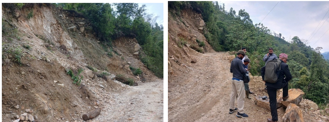
Photograph 3 Landslide Site, Bilaune Pakba
