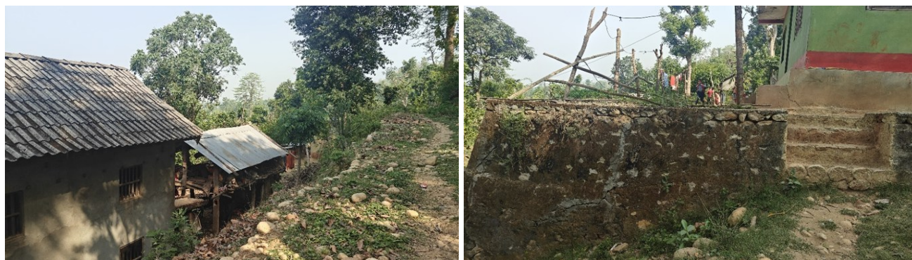
Photograph 80 Landslide Site, Bhedabari Mathillo Lamitale Tole
