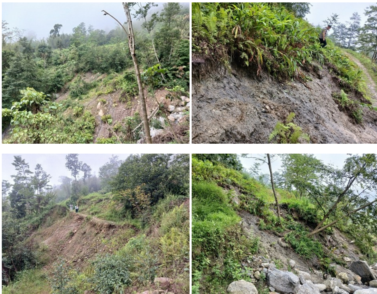
Photograph 28 Landslide Site, RongTol Khabare Khola Malim
