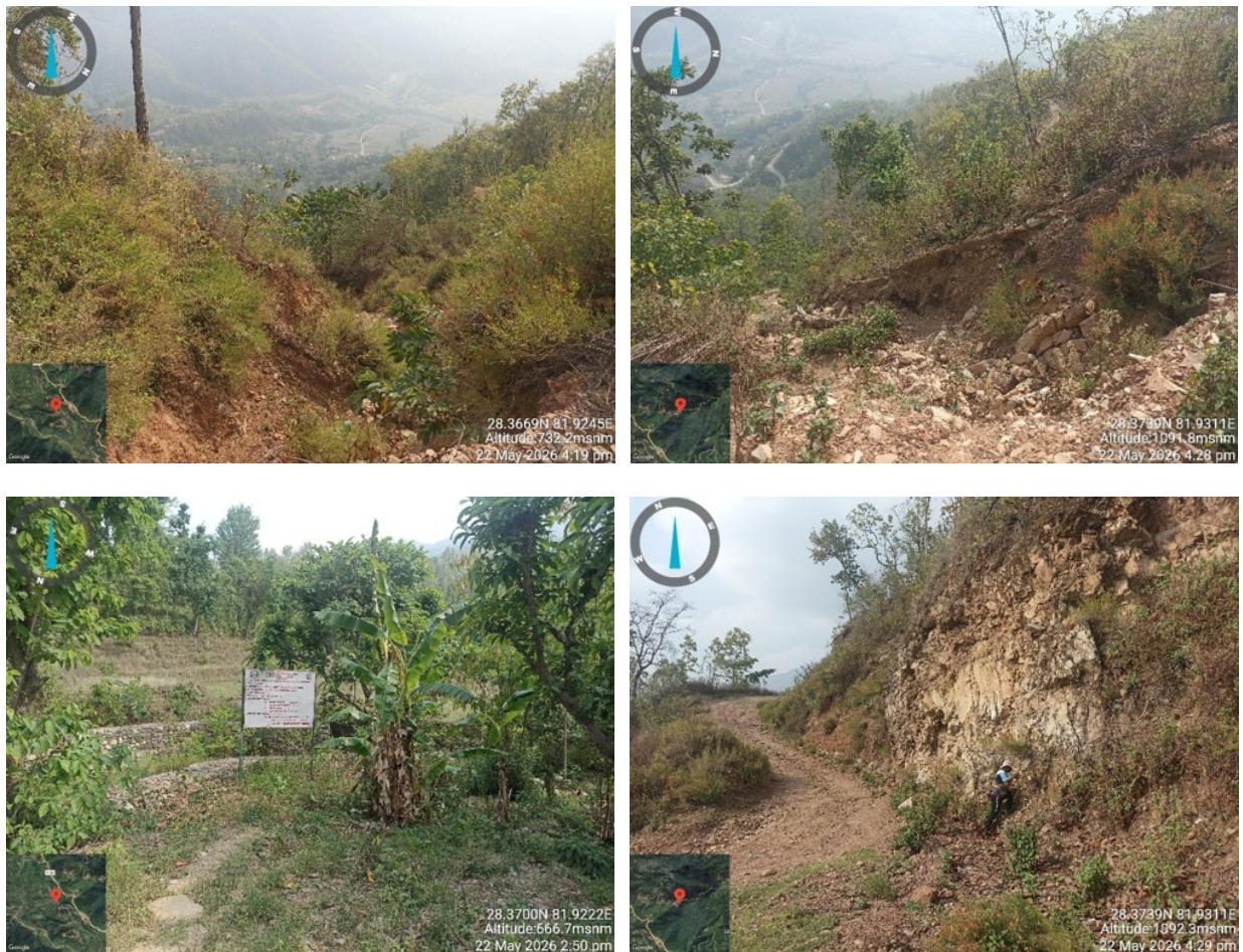
Photograph 62 Landslide Site, GhartiBase
