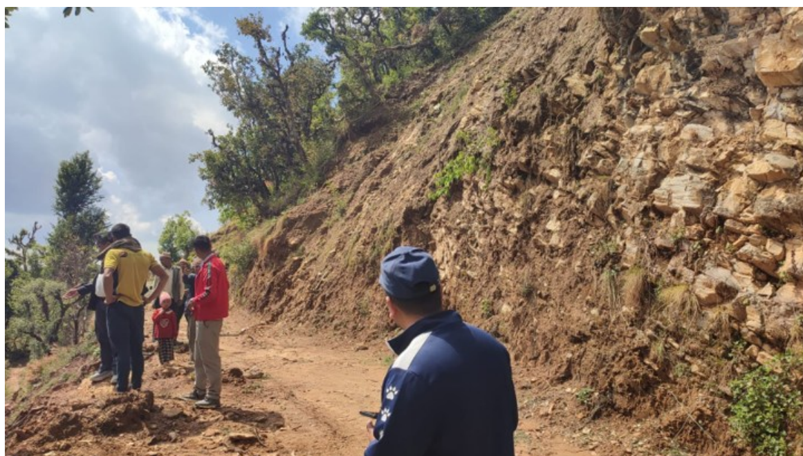
Photograph 60 Landslide Site, Chaura
