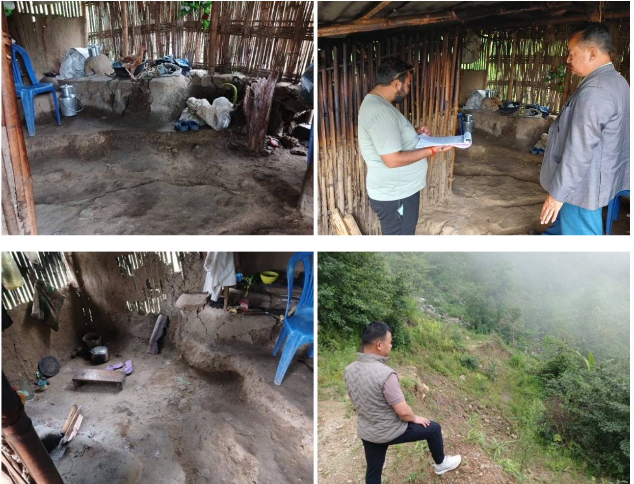
Photograph 34 Landslide Site, Lumke Tol
