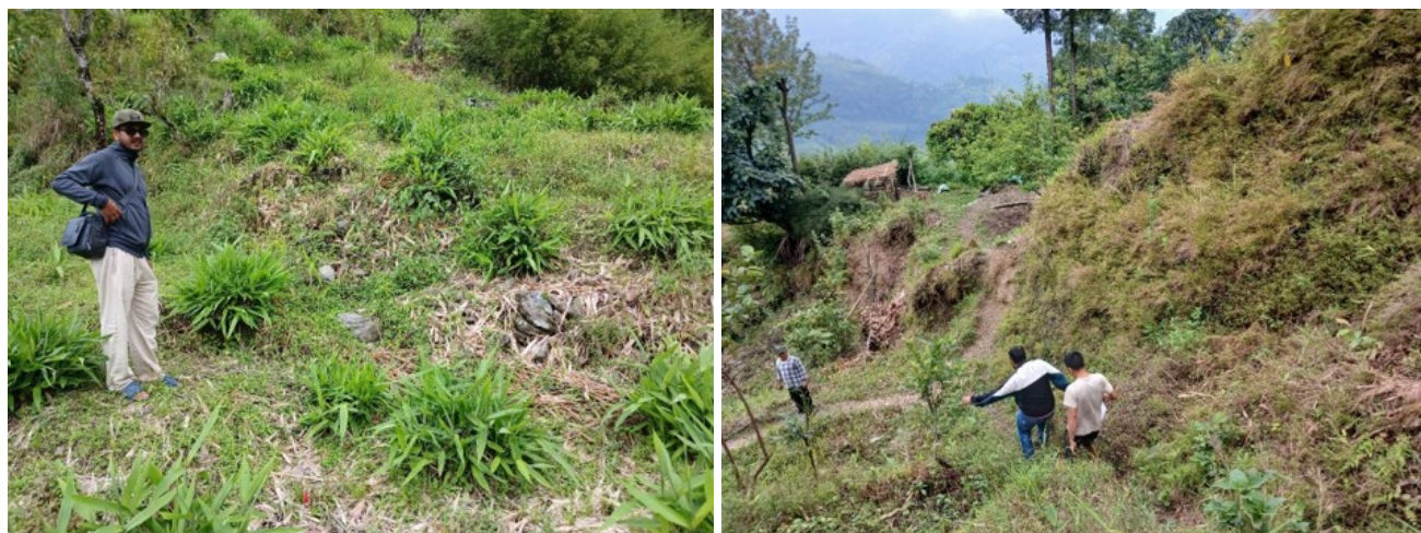
Photograph 23 Landslide Site, Ambe Tol
