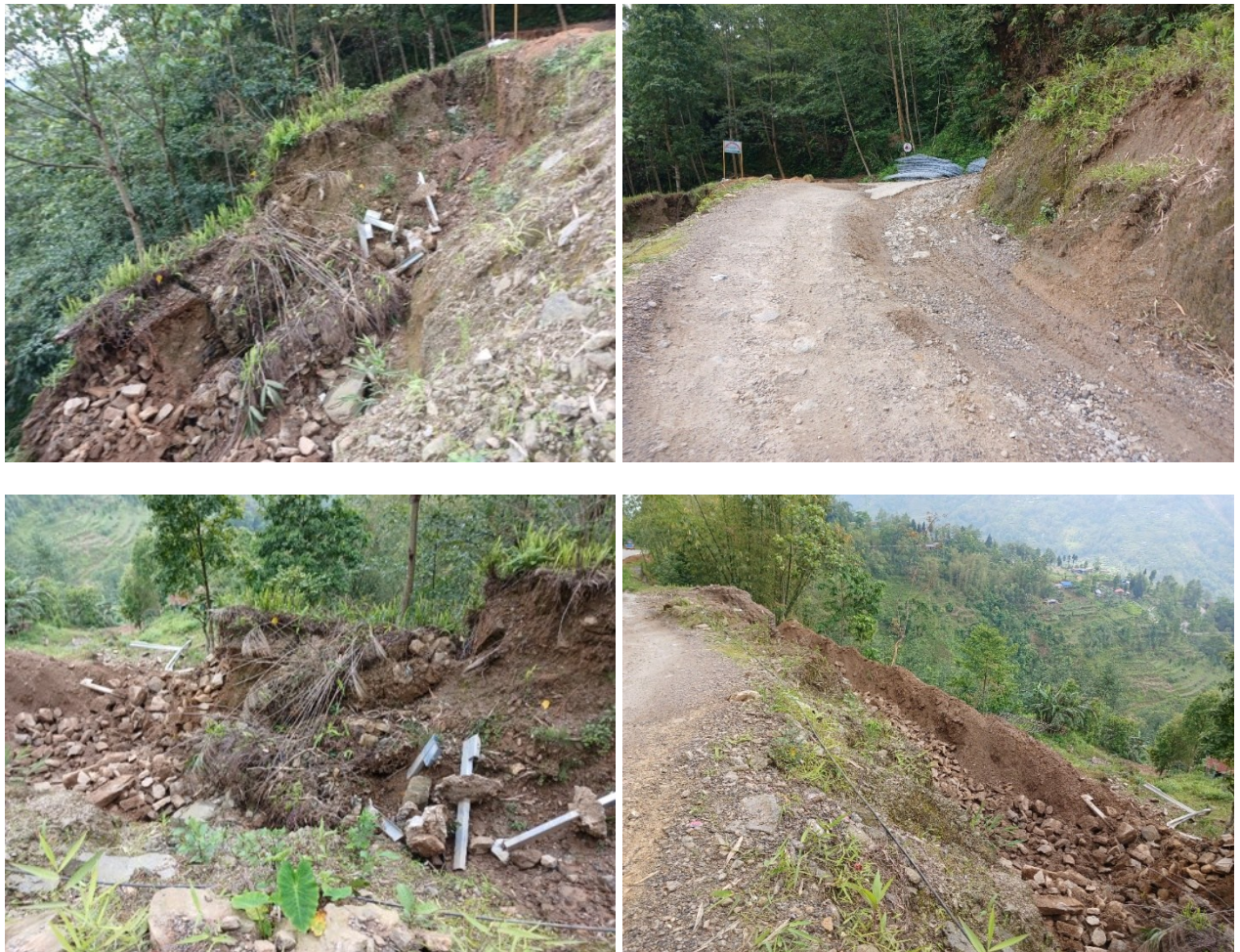
Photograph 24 Landslide Site, Dbode
