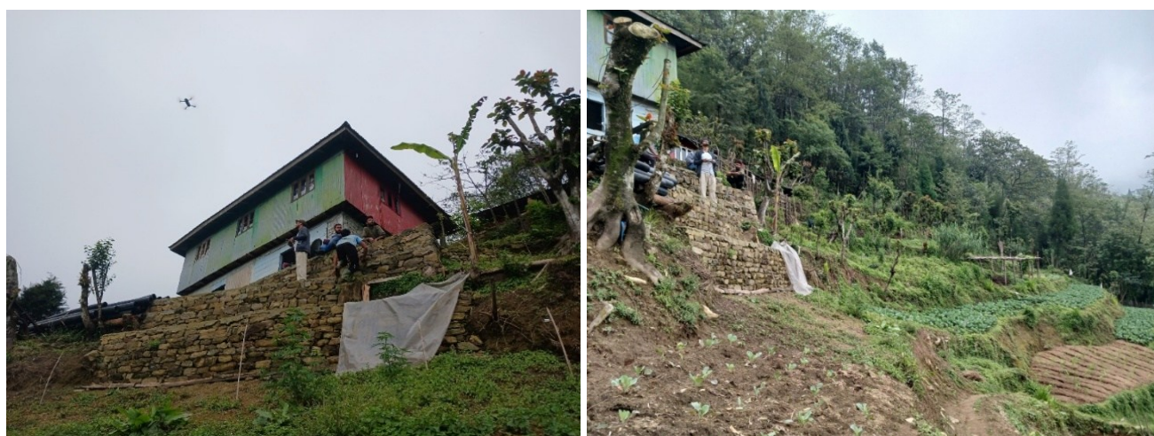
Photograph 2 Landslide Site, Shreekhola Chaghare
