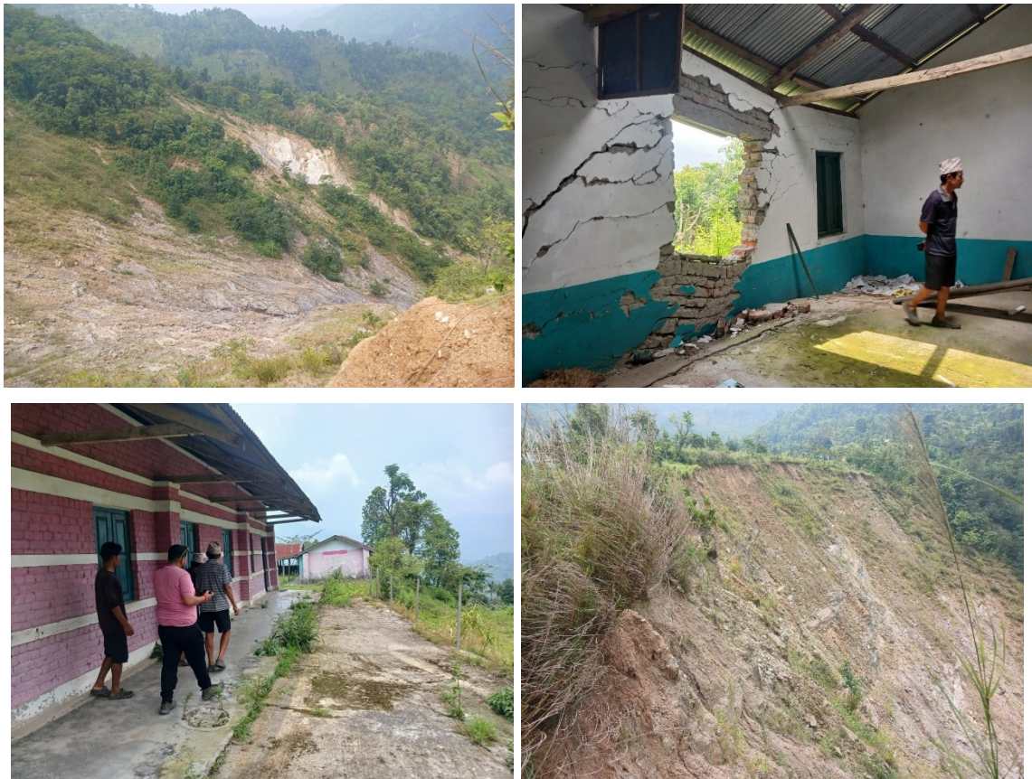
Photograph 40 Landslide Site, Rangapani
