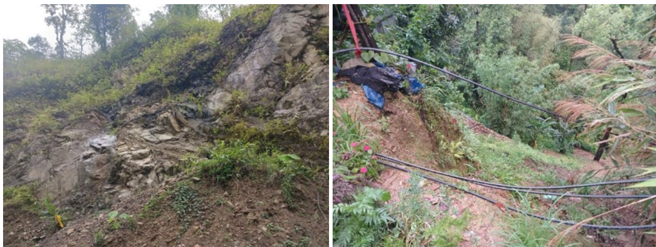
Photograph 48 Landslide Site, Bhanjyang
