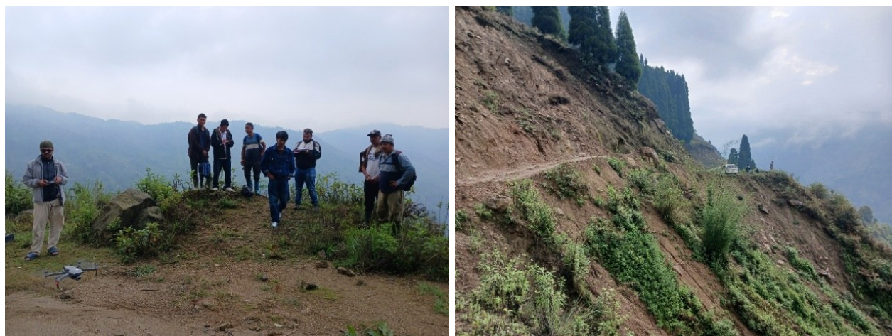
Photograph 6 Landslide Site, Chhaghare Jirel (Sagarmatha Tol)
