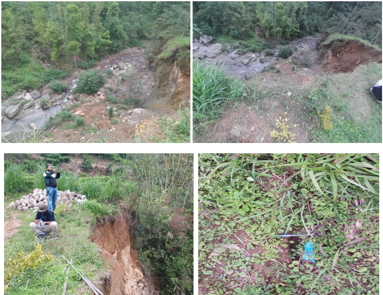
Photograph 9 Landslide Site, Siddhikboula Area
